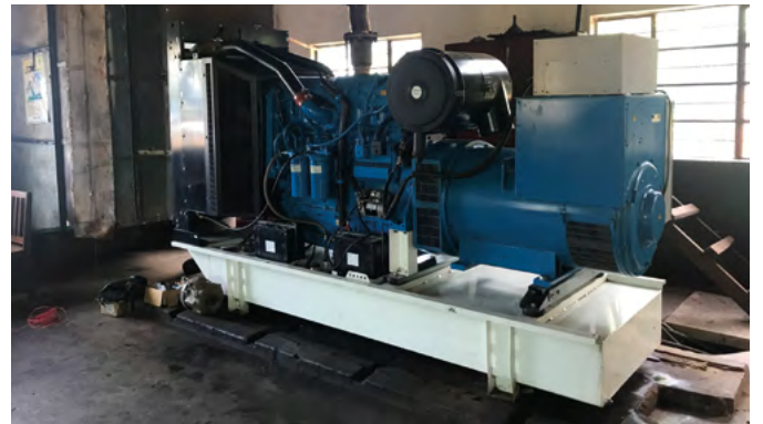
Diesel genset supplying a sawmill
